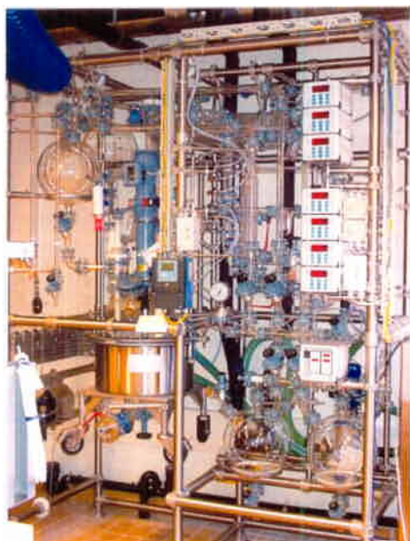
Fig. 4. Kilo lab is equipped with 30 l reactors (Büchi) and several smaller size glass reactors
